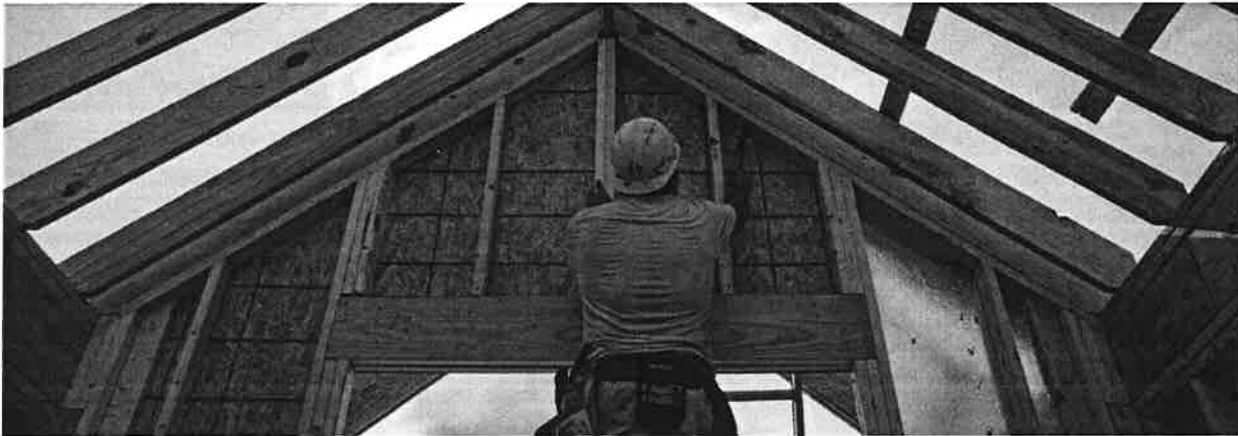
Workers build homes in Lillington, North Carolina, on June 15. Photographer: Allison Joyce/Bloomberg
